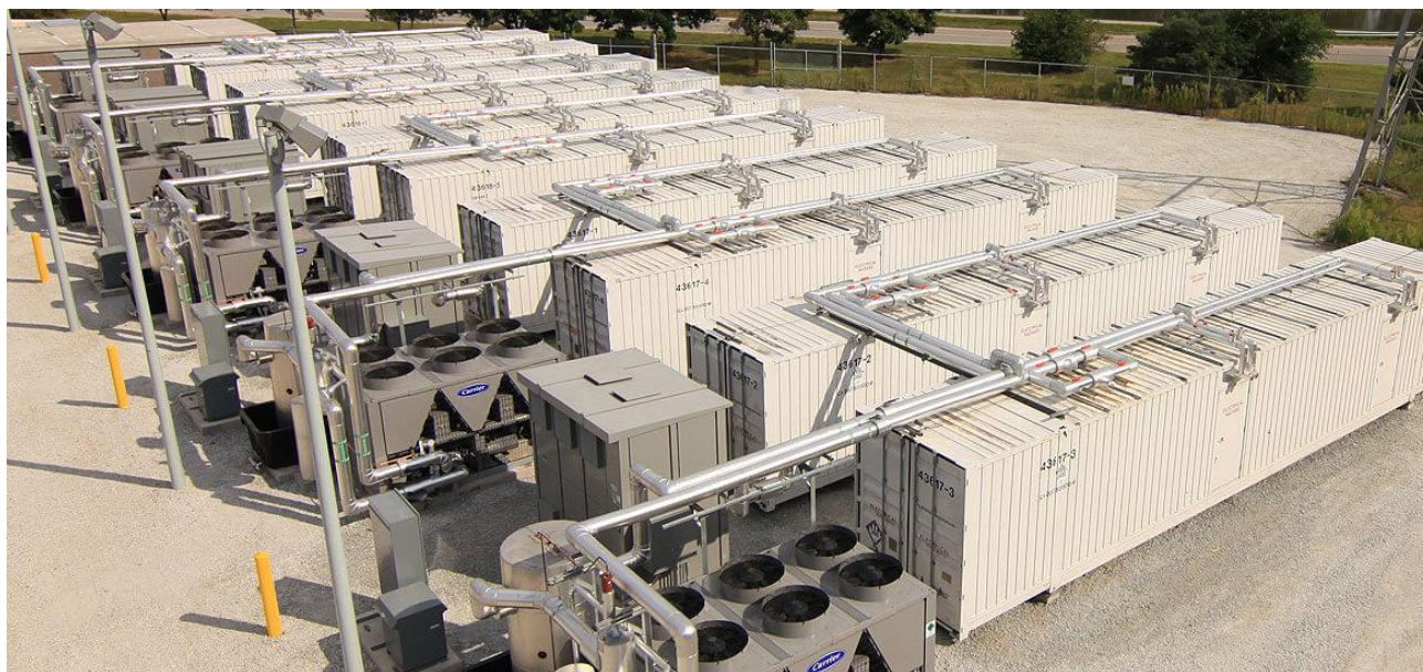
Figure 3: Typical containerized BESS facility (source: smart-energy.com)
